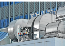
HVAC Air Compressor Pumps
